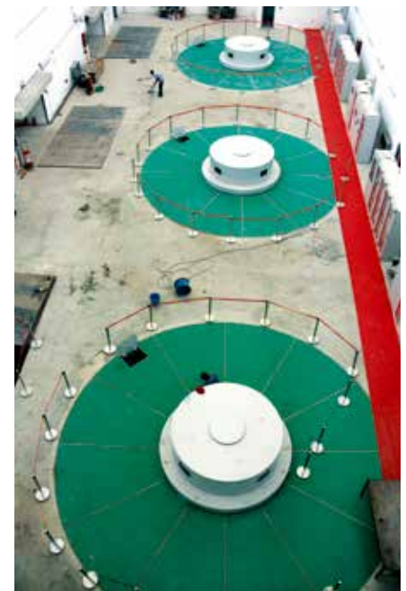
▲ Generating Units in Main Power House
